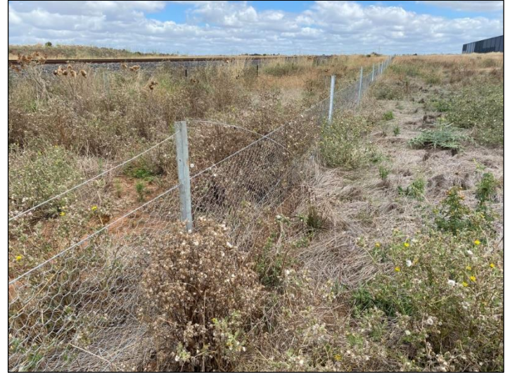
Plate B4.6. Broken wire in zone 2D (Ecology and Heritage Partners Pty Ltd 10/02/2022).
