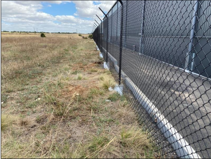
Plate B4.5. Cyclone fence installed post-installation (Ecology and Heritage Partners Pty Ltd 10/02/2022).
