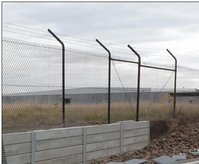
Plate A5.3. Rabbit proof fencing attached to cyclone fence, retaining wall and buried beneath rocks (Photo provided Citius 8/04/2022).
