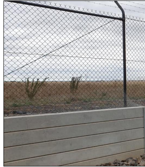
Plate A5.2. Rabbit proof mesh attached to the retaining wall and cyclone fencing (Photo provided by Citius 8/04/2022).
