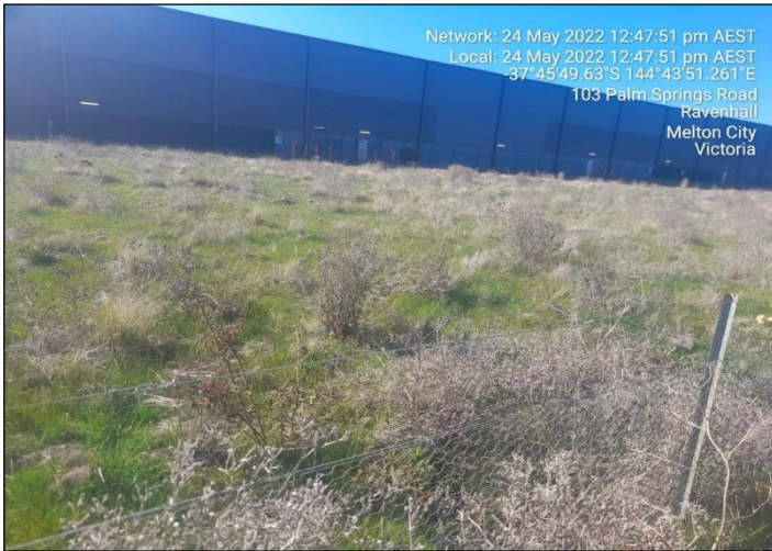
Plate A5.5. Repaired broken wire in zone 2D (Photo provided by Citius 25/05/2022).
